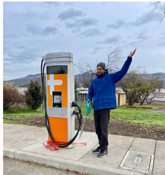
Michael Hoch stands next to an EV charging station installed as part of the City of Talent’s energy plan goals. Photo credit: City of Talent
